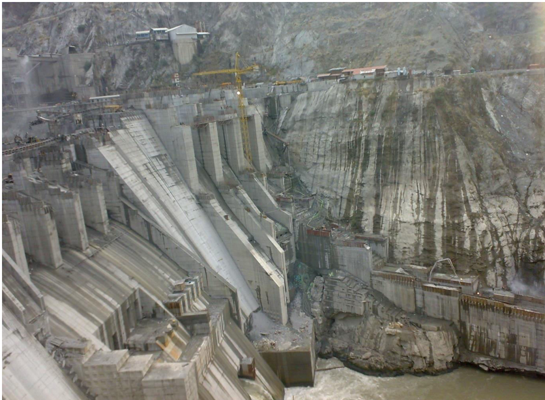
Baglihar Dam Hydroelectric Power Project is a run-of-the-river power project on the Chenab River in Jammu and Kashmir. It is based on the study of gravitational force, river profile and base level. This project is typical type of construction, built by Jaypee Group, India.
